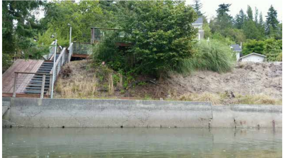
Our failing bulkhead prior to installing a "soft" shoreline.
